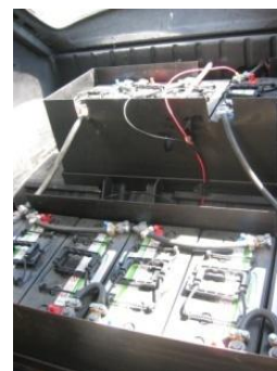
10 Advanced Glass Mat (AGM) lead- acid batteries
