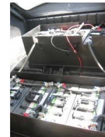
10 Advanced Glass Mat (AGM) lead-acid batteries
